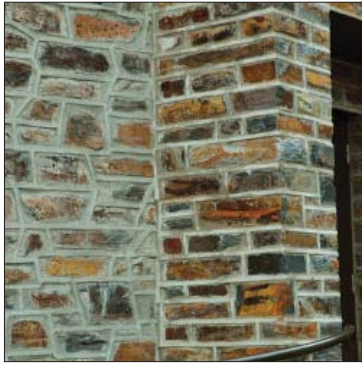
Duke Stone improper on the left and proper on the right
