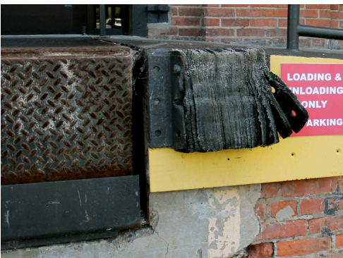
LOADING AREA Found on Smith Warehouse
